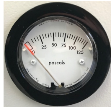
Figure 23: analog pressure display (manometer) for compressed air sweeping on the chamber front
