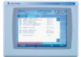
Alternate Local HMI Panel
