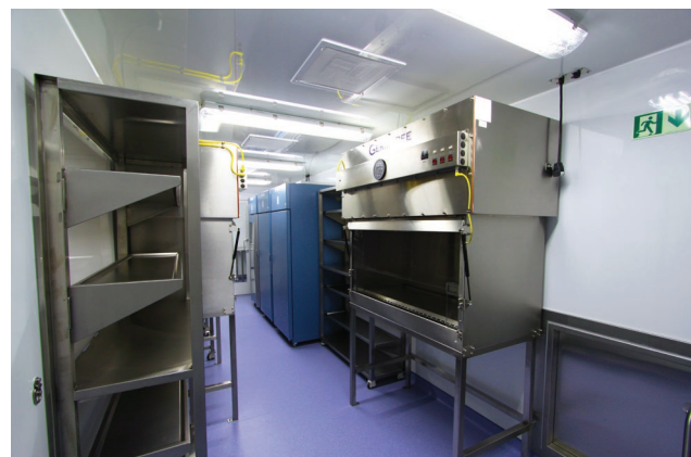
Class II, Type A2 Biological Safety Cabinet inside the Laboratory
