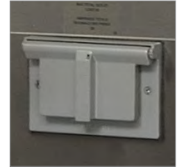
Duplex and/or GFI Outlets
