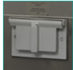
Duplex and/or GFI Outlets
